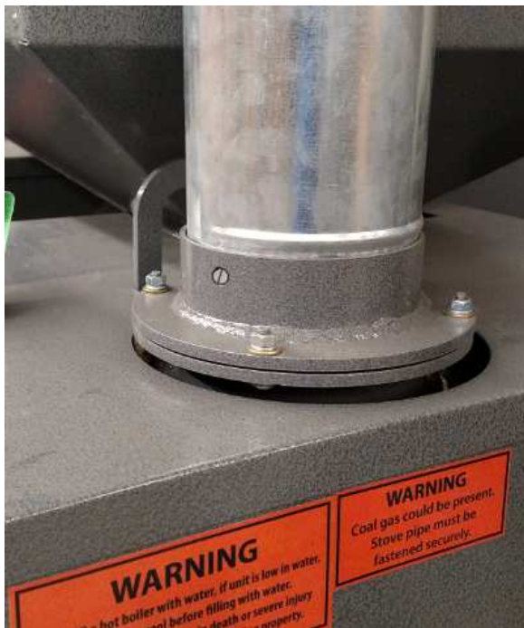
Flue Pipe Connection
