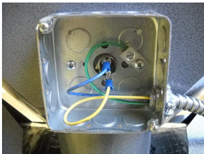
Hopper Temperature Safety Switch: Cover Open
