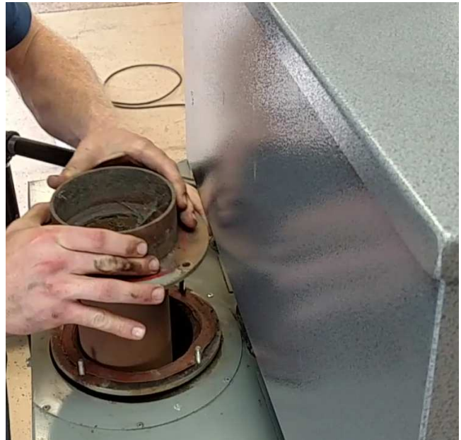
Lifting Out the Flue Tube Assembly
